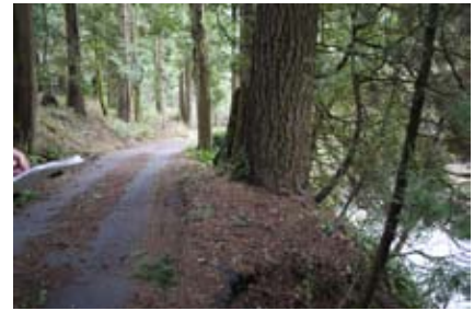
Figure 53: Tree adjacent to road on eroding bank
