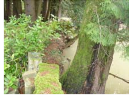
Figure 55: Tree growing from bank armoring
